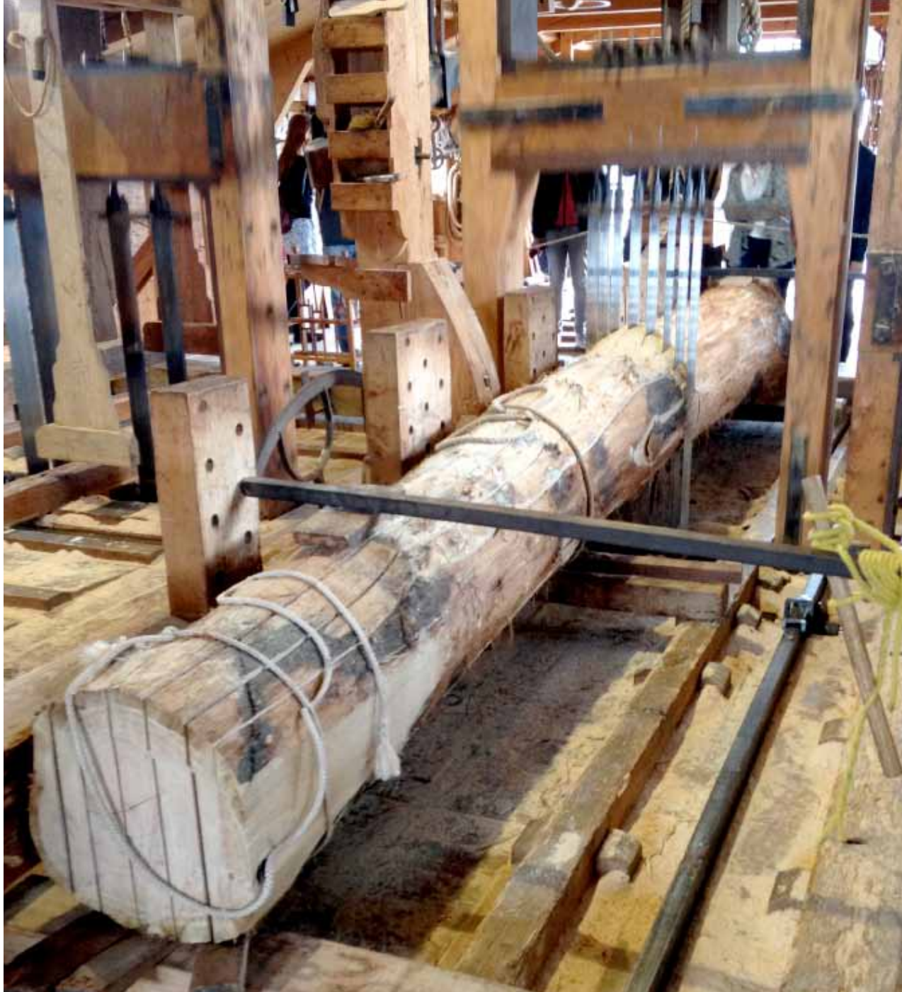
Facing page top: The fully restored Young Sheep today. Below: The sawmill has adjustable sawframes to cut planks with different thicknesses simultaneously. Above: On its saw carriage, the log inches through the saws at varying speeds dictated by the wind.
